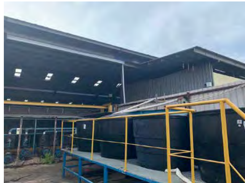
Rainwater Harvesting Used in Ijok Plant for Production.
